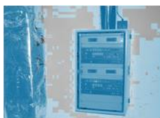
Remote Cabinet for Switchers and controllers
